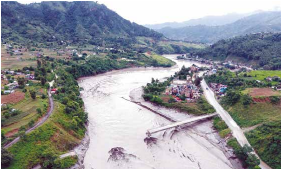
The damaged Ghatbesi Bridge over the Trishuli River in the aftermath of flash floods in Nepal's Dhading district
