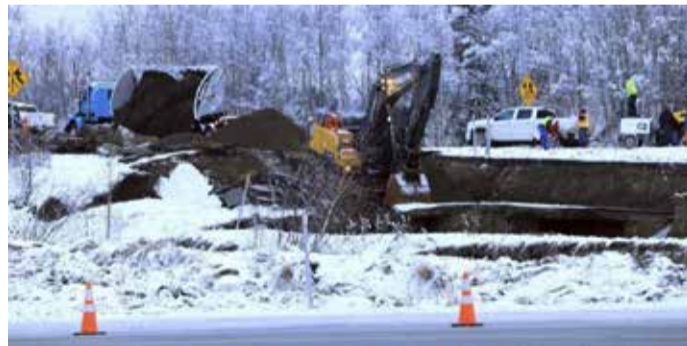
A dump truck and excavator work on a temporary fix of an off ramp that collapsed after an earthquake (file photo)
