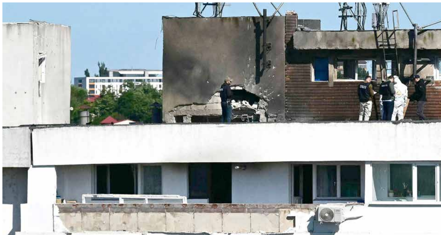
Police and forensic investigators stand on the rooftop as they examine the location of impact (C) over a damaged apartment
