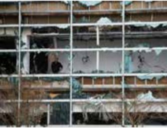
A damaged building in Louisiana
