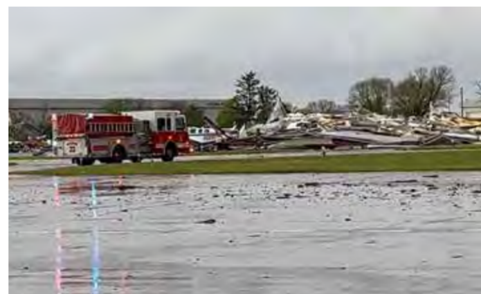
Emergency personnel work next to the damages caused by a tornado at Eppley Airfield, in Omaha, Nebraska
