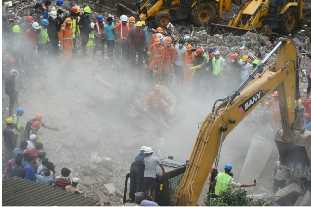
Rescue workers search for survivors in the rubble of the collapsed five-storey apartment building in Mahad
