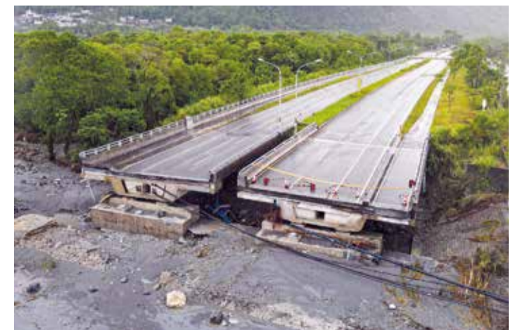
Part of the bridge over Mataian Creek is seen damaged after a barrier lake burst in Hualien
