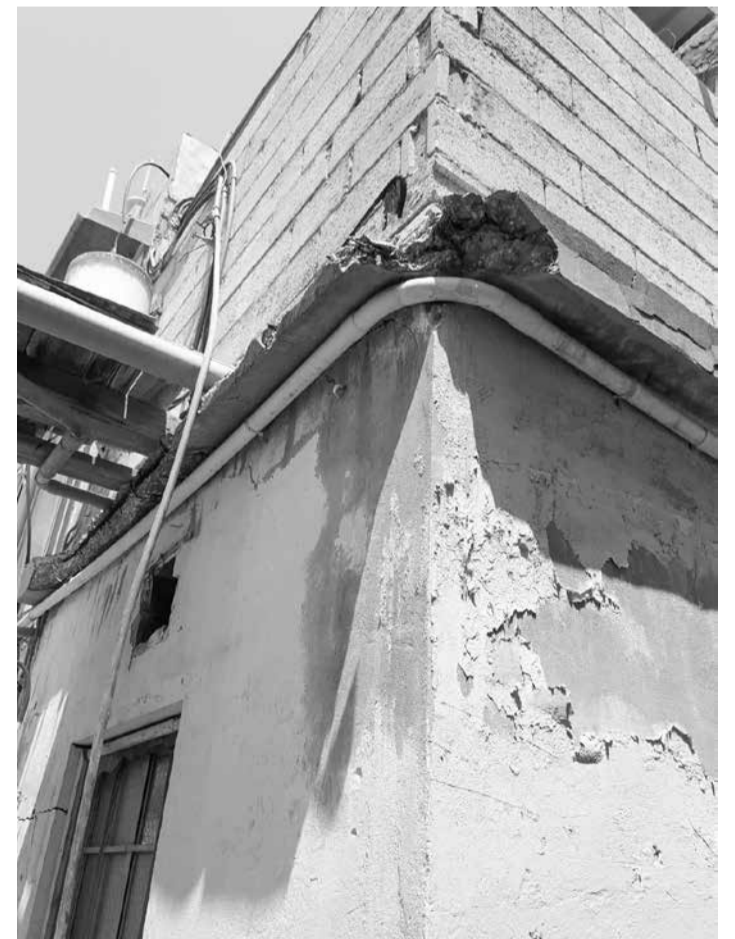
The house can collapse anytime.
