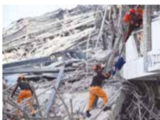
Twenty people were listed as missing after the collapse of the nine-storey building under construction in Angeles City
