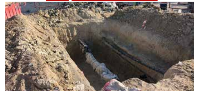
The Ministry of Works' project to develop the intersection of Street 46 with Al Hidd Street and Road No. 4338 in Block 243 in Arad has reached 70%. It aims to improve the efficiency of the public street network and increase its capacity.
