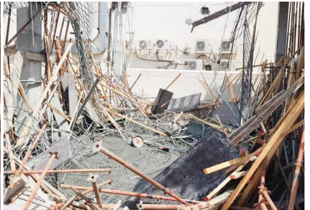
The remnants of the structure that collapsed.
