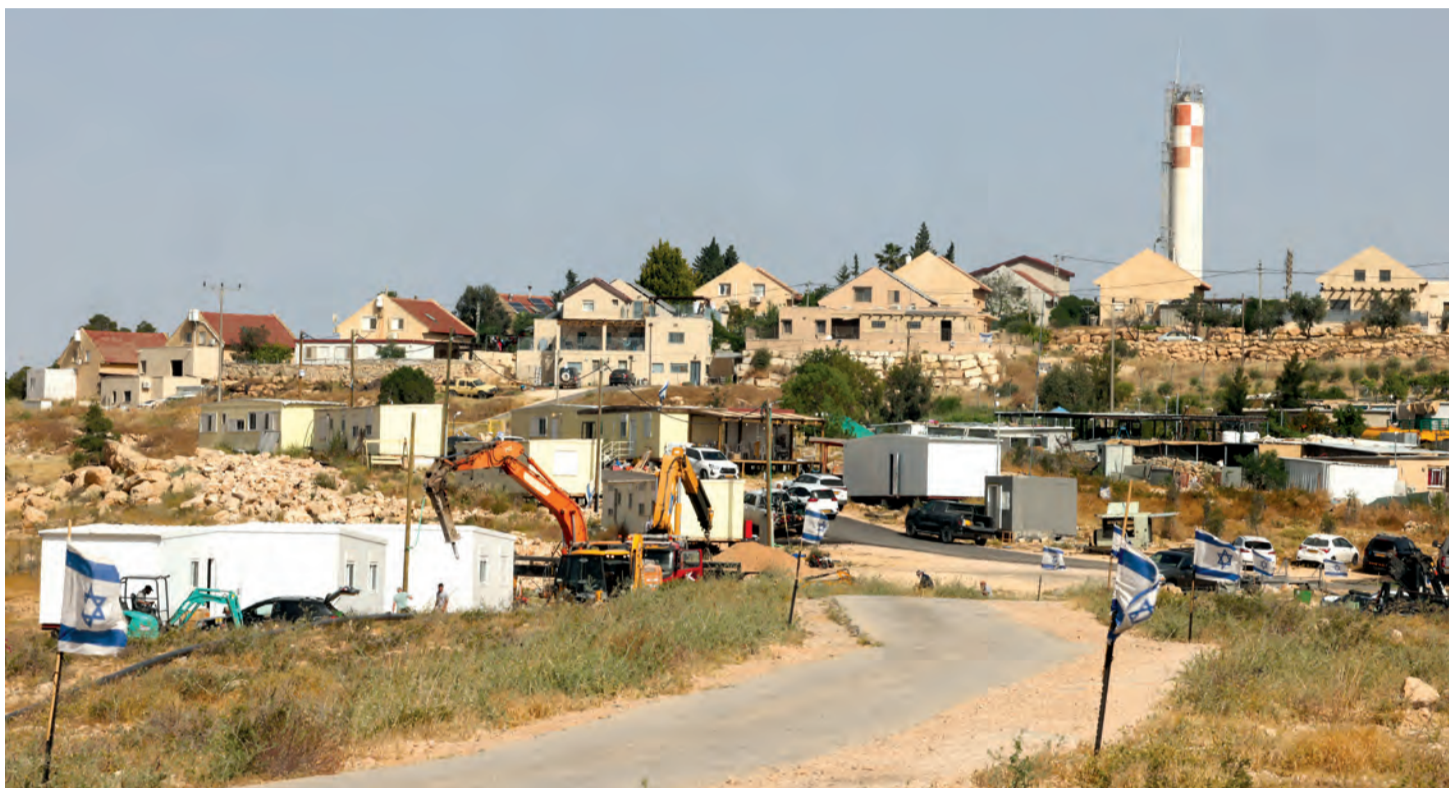
New prefabricated Jewish outpost homes are placed in position along a road that heads toward the Palestinian village of Umm al-Khair, wedged between the new outpost of Karmel (foreground Left) and the Israeli settlement of Karmel (hilltop), south of the town of Yatta in the southern area of the Israeli-occupied Palestinian West Bank
