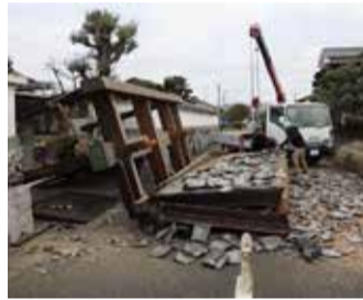
A collapsed gate to the residential house caused by an earthquake is seen in Oita, southern Japan
