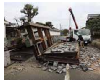
A collapsed gate to the residential house caused by an earthquake is seen in Oita, southern Japan
