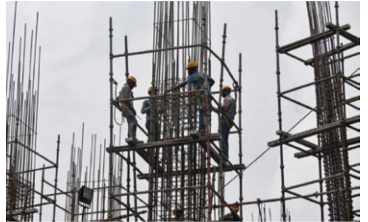
Workers erect scaffolding at a construction site of a metro rail station in Kolkata, India
