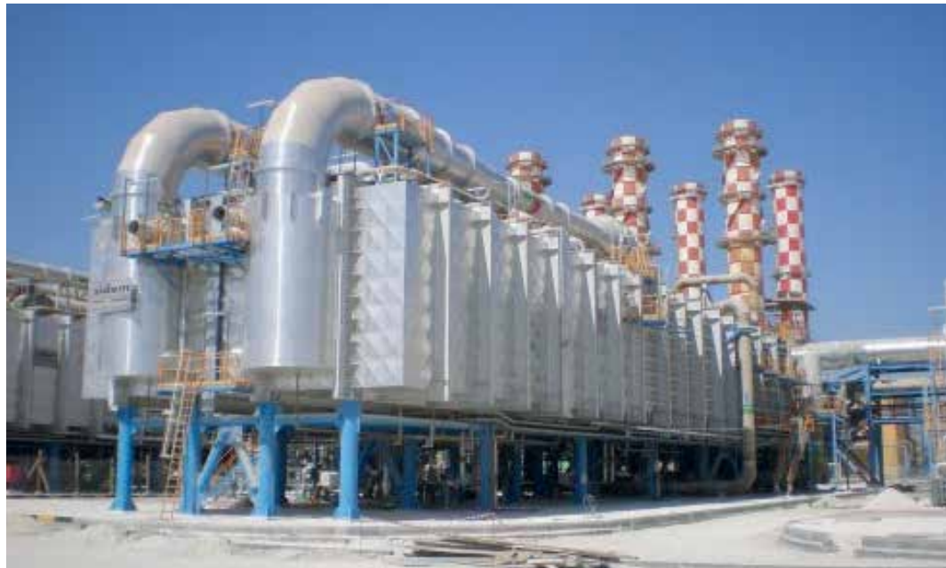
A desalination plant in Al-Hidd
