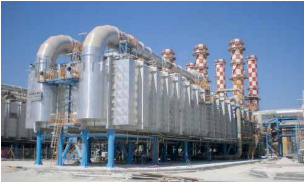
A desalination plant in Al-Hidd
