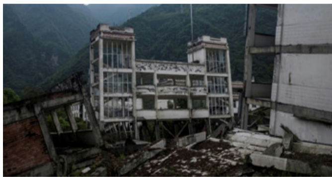
This picture taken on April 21, 2018 shows part of the destroyed Xuankou Middle School, now the memorial site for the 2008 quake
