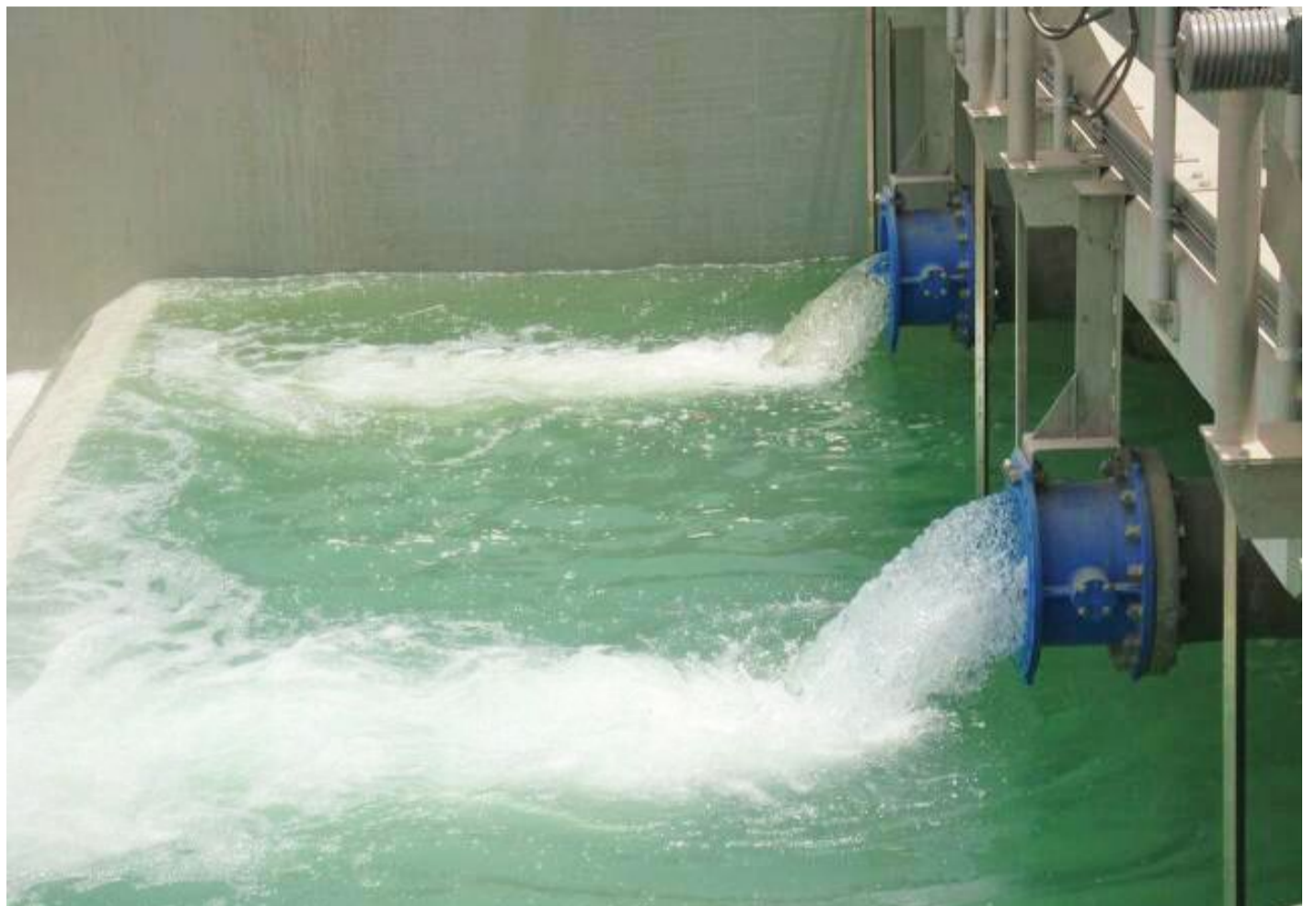
Seven hundred farms directly benefit from the Tubli Wastewater Treatment Plant.
