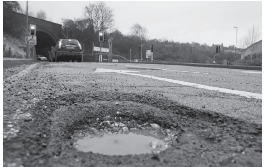
In the UK, more than 3,000 bridges were found not fit to carry the heaviest vehicles (Representative picture)
