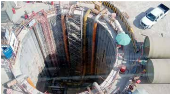
The new line connects the assembly room of the main lines and pumping station
