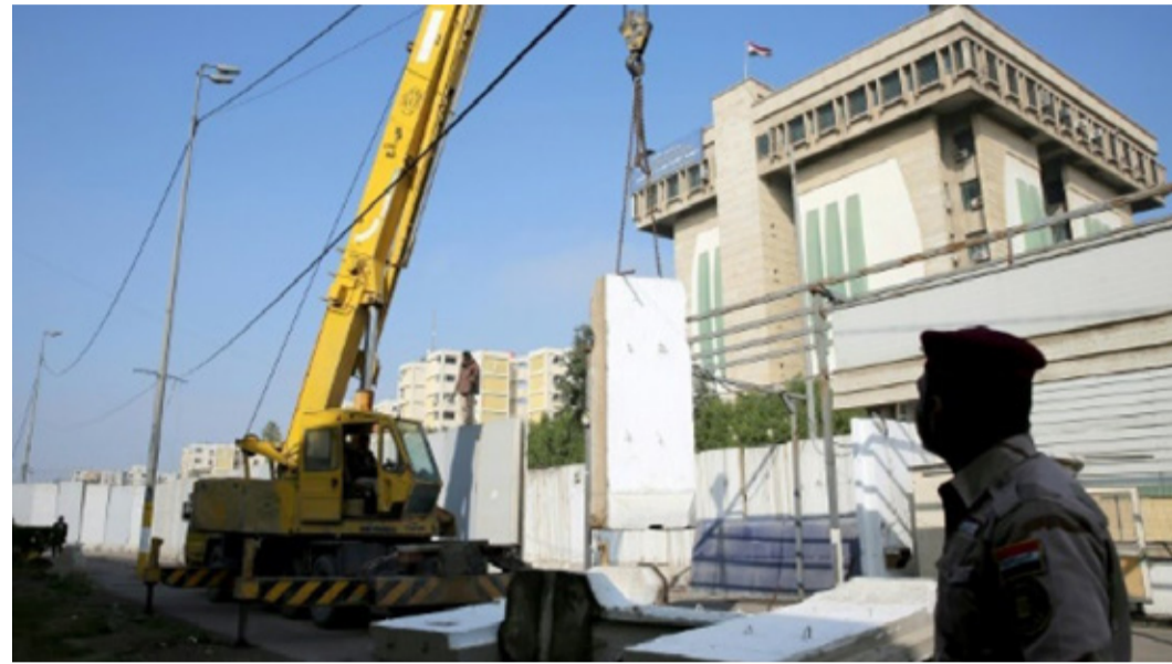
Workers remove cement blast walls surrounding the Iraqi foreign ministry near Baghdad's Green Zone
