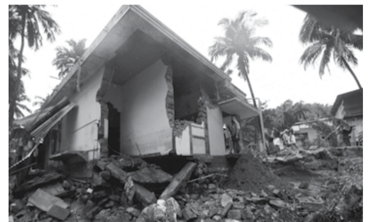
Local residents look at a partially destroyed house after heavy monsoon rains led to a landslide in Kannappankund, in the Indian state of Kerala
