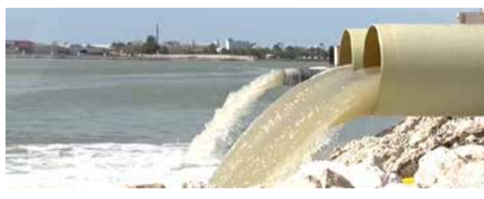
The Ministry of Municipalities and its supporting teams are working on sucking rainwater from the region and its streets and pumping it to Lake Al-Luzi
