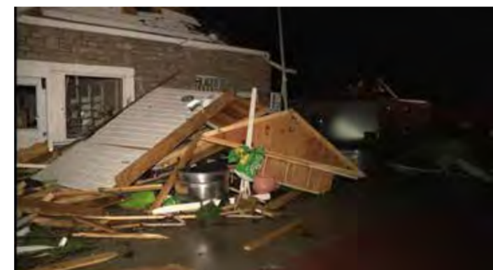
Damage from tornadoes that ripped through Indian Lakes
