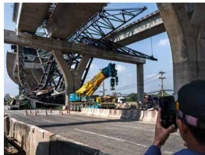
A recovery worker takes pictures at the site of a construction crane collapse
