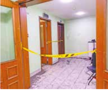
Fire-hit Al Ramli flat sealed off after the August 18 family tragedy
