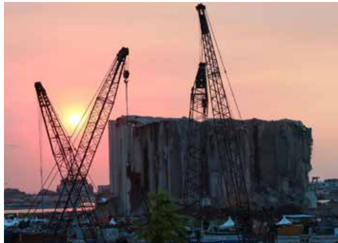
A view shows the grain silo that was damaged during last year's Beirut port blast, during sunset in Beirut, Lebanon,
