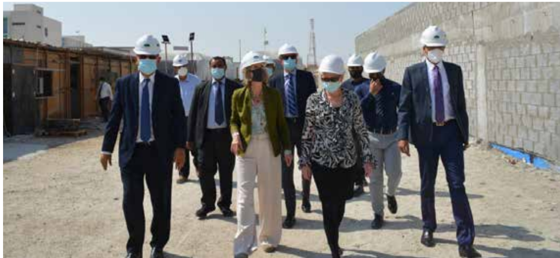
US Embassy charge d'affaires Margaret Nardi paid a visit to the ongoing construction site of the King Hamad American Mission Hospital in A'ali. Nardi was given a tour and shown around the site by AMH Corporate CEO Dr George Cheriyan and Group CEO Julia Tovey.
