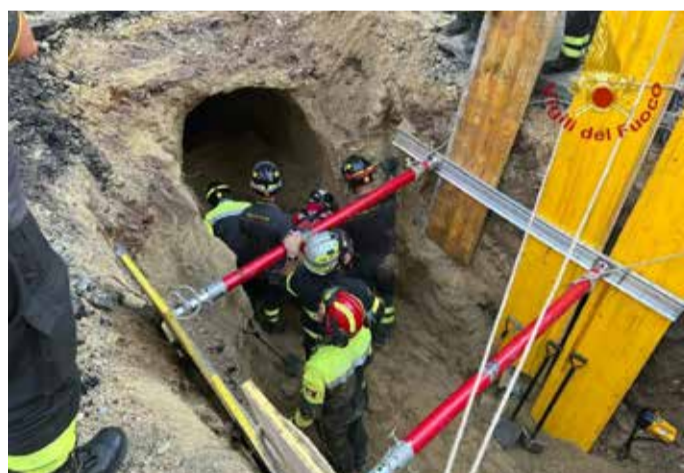
First responders during a rescuing operation for a suspected thief who was buried under rubble for about eight hours, as he was allegedly digging a tunnel with his accomplices
