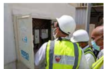
Team members check on the safety of electricity connections at one of the shared accommodations
