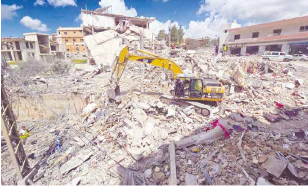
An excavator clears the rubble of destroyed buildings from the site of an Israeli strike that targeted the southern Lebanese village of Qana
