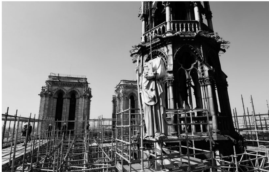
One of 16 copper statues, sitting 50 meters above the ground, is lifted off the Notre-Dame-de-Paris Cathedral to be taken for restoration on April 11, 2019 in the French capital Paris.
