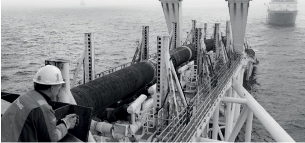
A man standing on the pipe-laying ship "Audacia" looking on as tubes are laid for the "North Stream 2" gas pipeline off the coast of the Baltic Sea island Ruegen, northeastern Germany.
