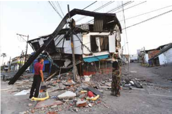
A couple stands amid the rubble of a collapsed house after an earthquake in Pereira, Colombia
