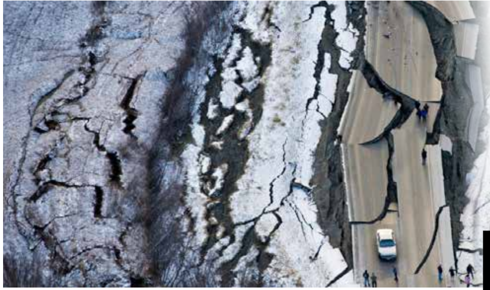
A damaged road is seen after an earthquake. (Representative picture, courtesy of Columbia Journalism Review)
