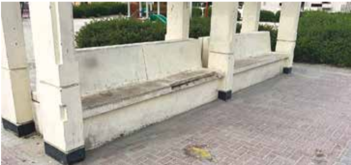
Public park benches need maintenance to ensure cleanliness
