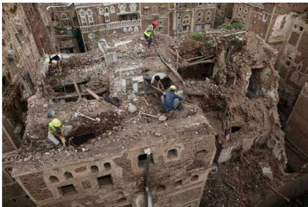
Workers demolish a building damaged by rain in the UNESCO World Heritage site of the old city of Sanaa, Yemen
