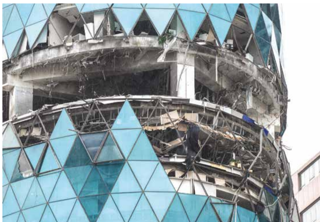
Damage to a building in Seef following an Iranian drone strike at dawn. (AFP)
