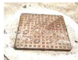
A manhole creates navigation challenges for pedestrians
