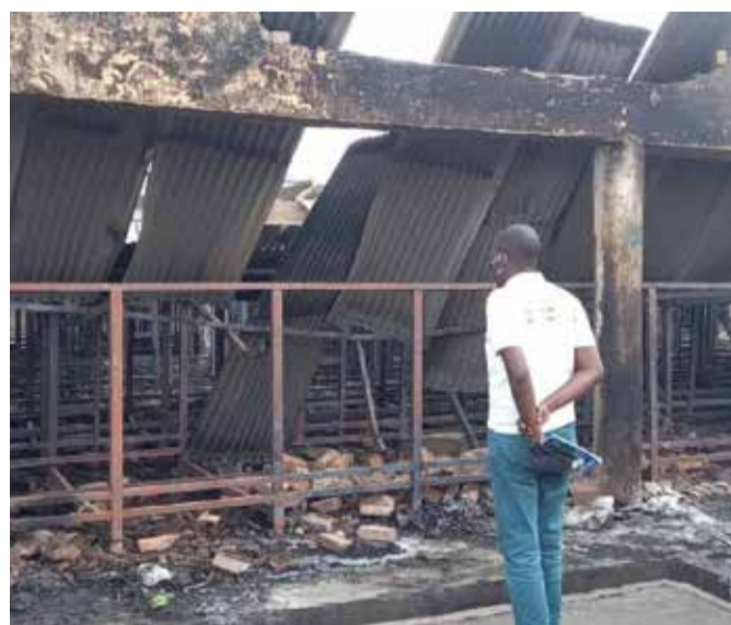
A journalist, policeman and a soldier observe the damage in front of the main prison after the fire, in Gitega, Burundi
