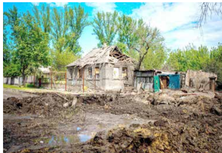
A photograph shows a damaged building after a missile strike in the town of Kramatorsk, Donetsk region (file photo)
