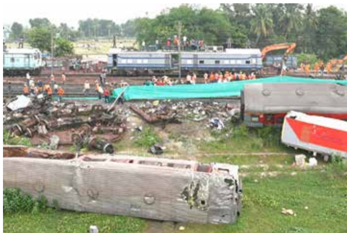
Railway workers help to restore services at the accident site of a three-train collision near Balasore
