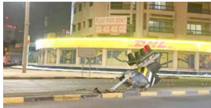
A broken traffic signal in Um Al Hassam
