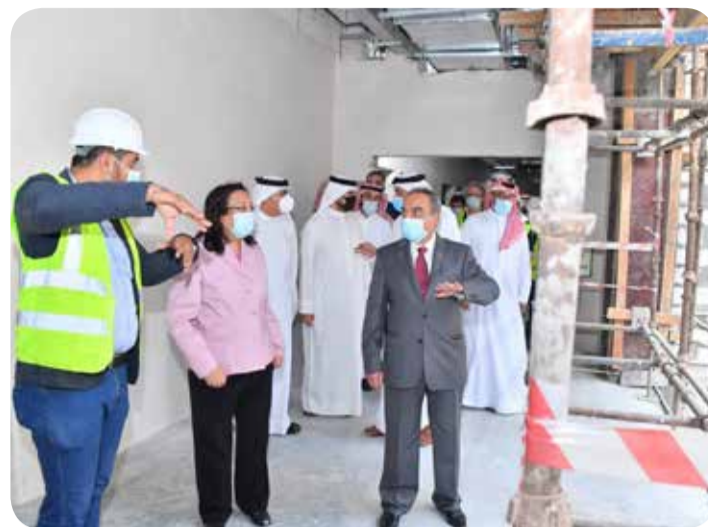
Essam Khalaf, the Minister of Works, Municipalities Affairs and Urban Planning and Faeqa bint Saeed Al-Saleh, the Minister of Health visiting the project site
