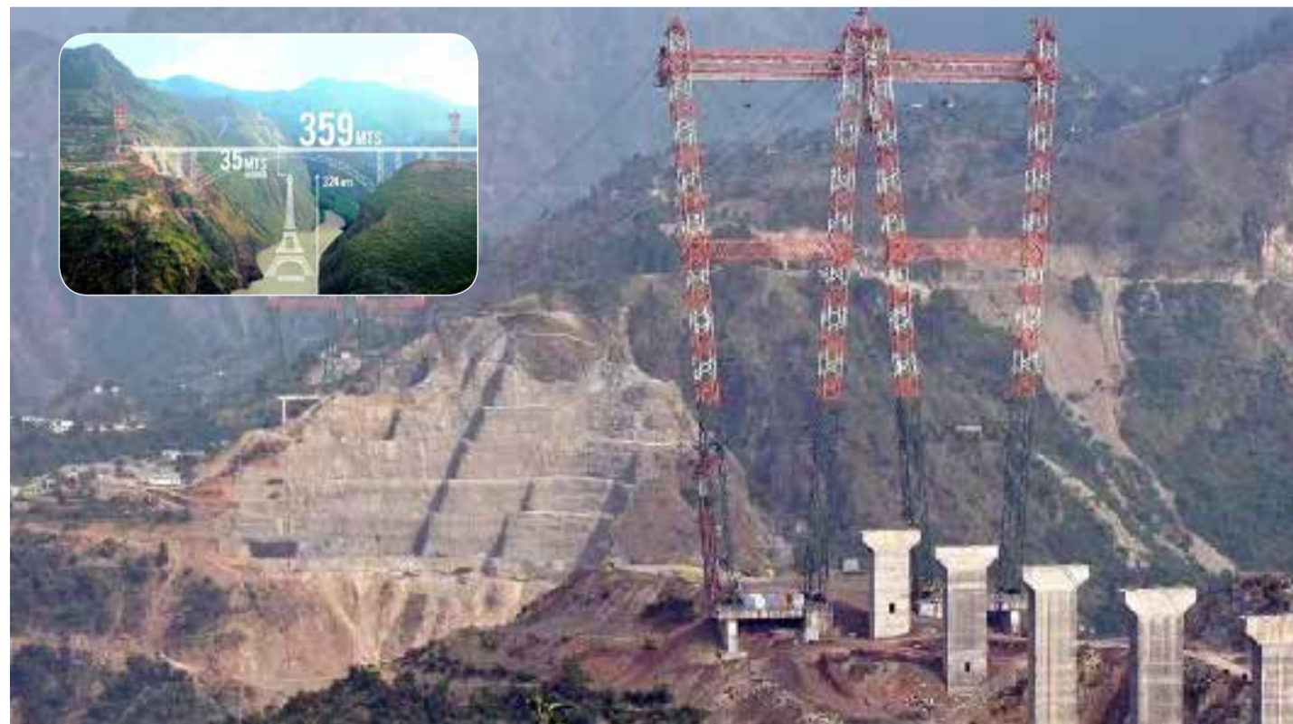
File photo of a general view of the site of the under-construction railway bridge on Chenab river in Jammu-Kashmir (HT /AFP File Photo ) Inset picture, courtesy of metrorailnews
