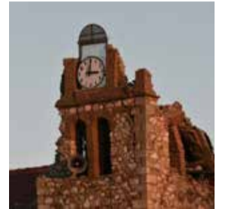
A church damaged in the quake
