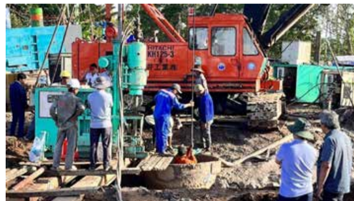
Efforts to rescue a Vietnamese boy trapped inside a hollow pillar at a construction site appear to have failed
