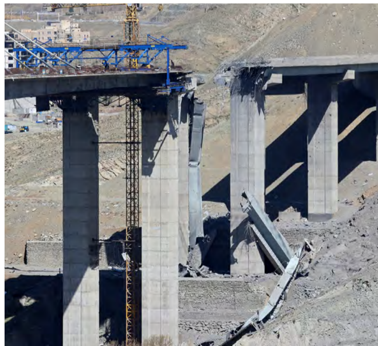
A view of the B1 bridge is pictured, a day after it was destroyed by a strike in Karaj
