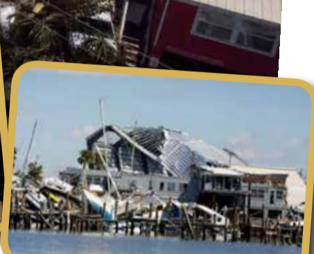
A destroyed marina in the Matanzas Pass
