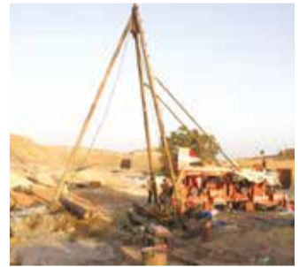
A view of work around an 84-metre well being dug to draw seawater
